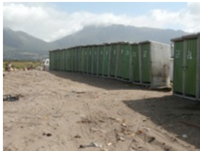
The toilets of the old TRA site they had to walk to before they broke the locks at the new TRA site. Each four households have a key to one toilet. The stench in the area, due to waste is unbearable.
